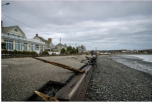
Damage to the seawall on Gooch's Beach in Kennebunk, Maine, is seen after a nor'easter battered the coast in early March 2018. Jonathan Bryant
