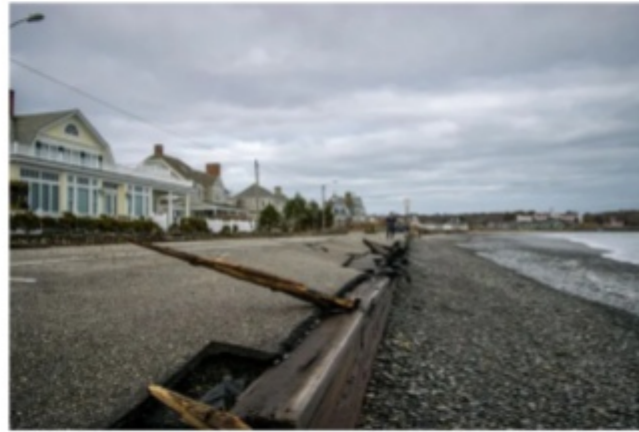
Damage to the seawall on Gooch's Beach in Kennebunk, Maine, is seen after a nor'easter battered the coast in early March 2018. Jonathan Bryant
